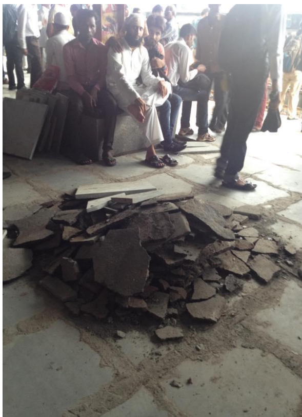
Hazardous Construction at Borivali Station
