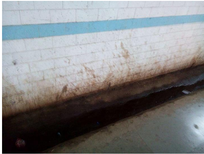
Hazardous & Unhygienic Subway at Dahisar
