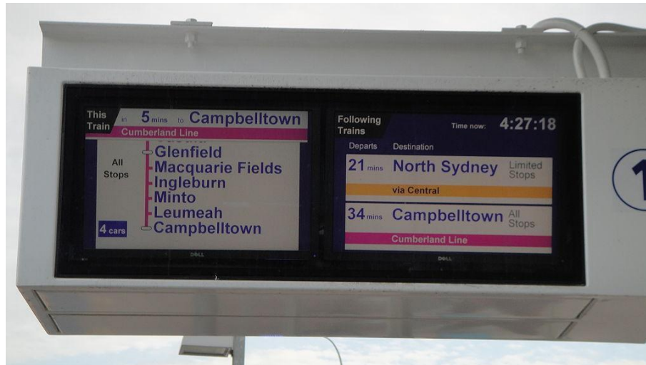
Platform indicators on all Sydney train platforms
